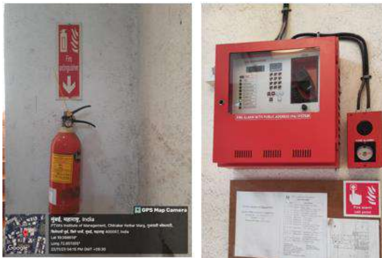
Fire extinguishers & Alarm Panel
