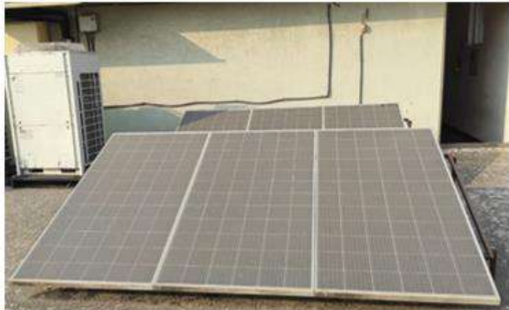
Solar Power System
