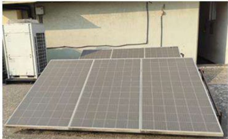
Solar Power Plant
