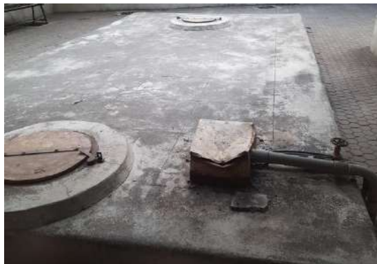
Rainwater Harvesting Pits
